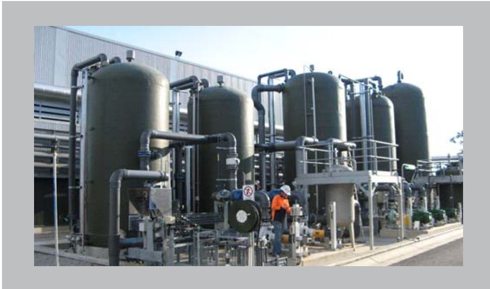
Figure D-3. Chemical Storage Tanks
